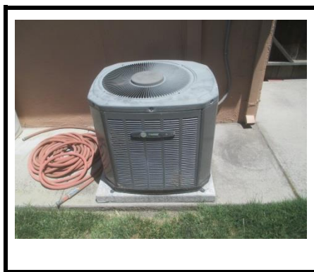
Picture 1... The A/C condenser was in acceptable working condition.
